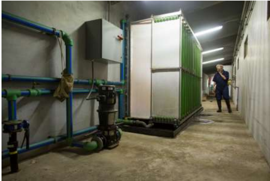
Figure 3. One of three geothermal heat exchangers or radiators that transfers energy from the geothermal system to the incoming air of 4 of the 16 rooms in the grow-finish barn.
