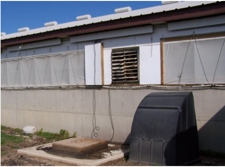
Figure 4. Pit fan has been move to sidewall.
