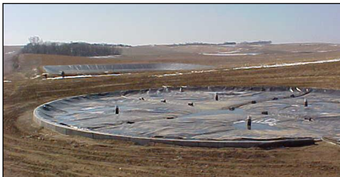
Figure 1. Digester and storage basin on study farm. (Photo by R. Stowell)
